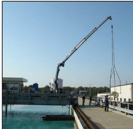
Using a crane, the ECO-Auger™ was positioned in the tank, then mounted below the main bridge and towed through the water.
