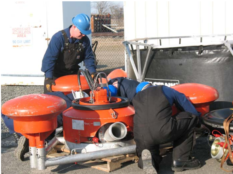
Figure 3: Station 2 – Pumping/Skimming Station (Fast Tank – 1K gallon)
