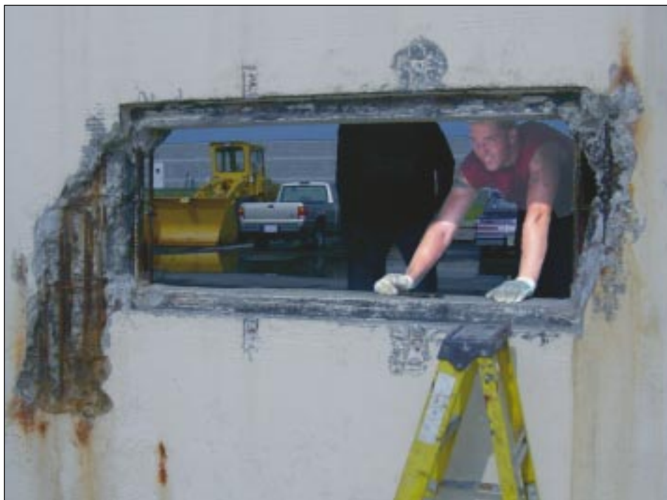
A technician peers through the gaping hole left when the old basin viewing window was removed.
