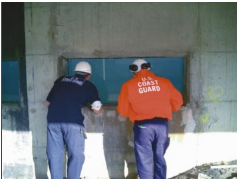
U.S. Coast Guard strike team members look through the new viewing window.
