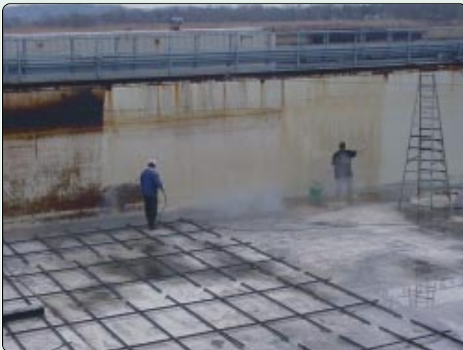
The test basin is emptied of water so Ohmsett staff can make repairs and clean the tank walls.
